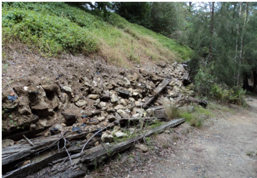
Photo 4 – Damaged timber retaining structures
