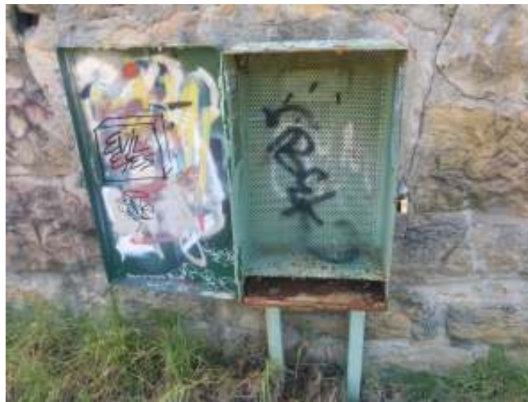
Photo 6 – Electrical box on lower bowling green
