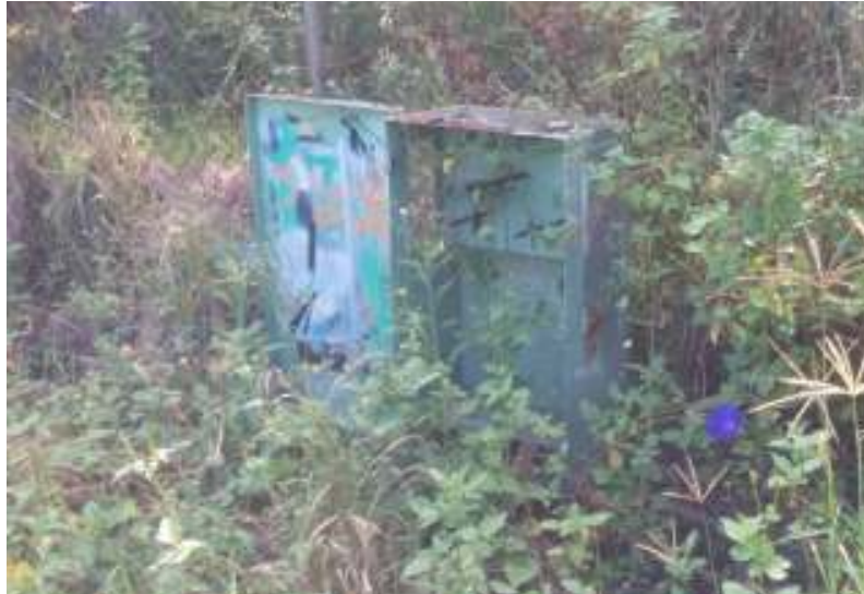
Photo 7 – Electrical box on upper bowling green
