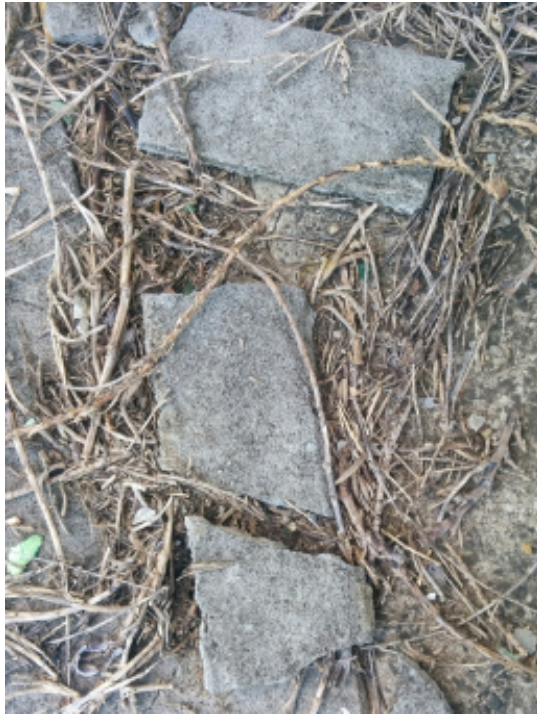
Photo 11 – Potential Asbestos Containing Material
